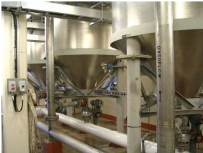
Sludge pre-pasteurization vessels
