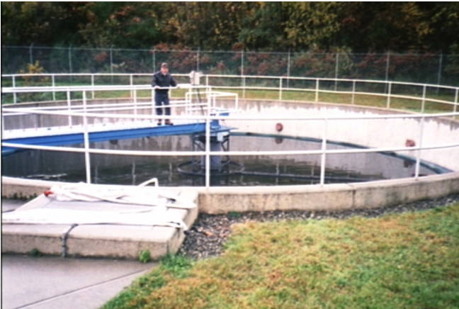
A secondary clarifier at the Windsor, VT, WWTF. Clarifiers mimic the conditions in a still pond, allowing solids to settle to the bottom where they are removed by a slowly-rotating scraper. These solids are then treated to become biosolids.
