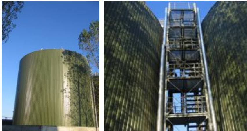
Multi-Feedstock BioGas plant Customer: SARIA ReFood
