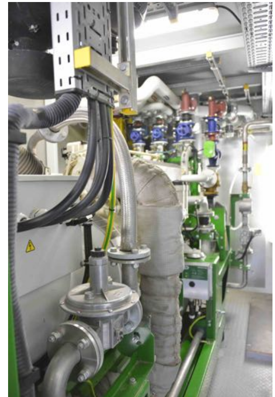
New engine at Essex Junction WWTF.
