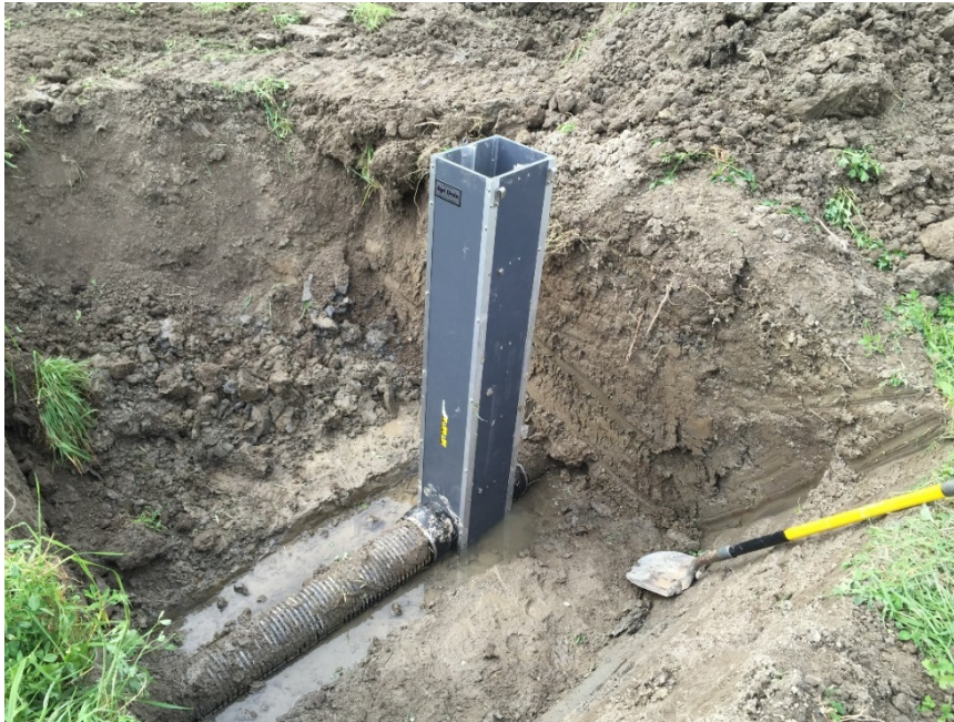
Figure 8. Agri-Drain water level control structure installed on tile drain
