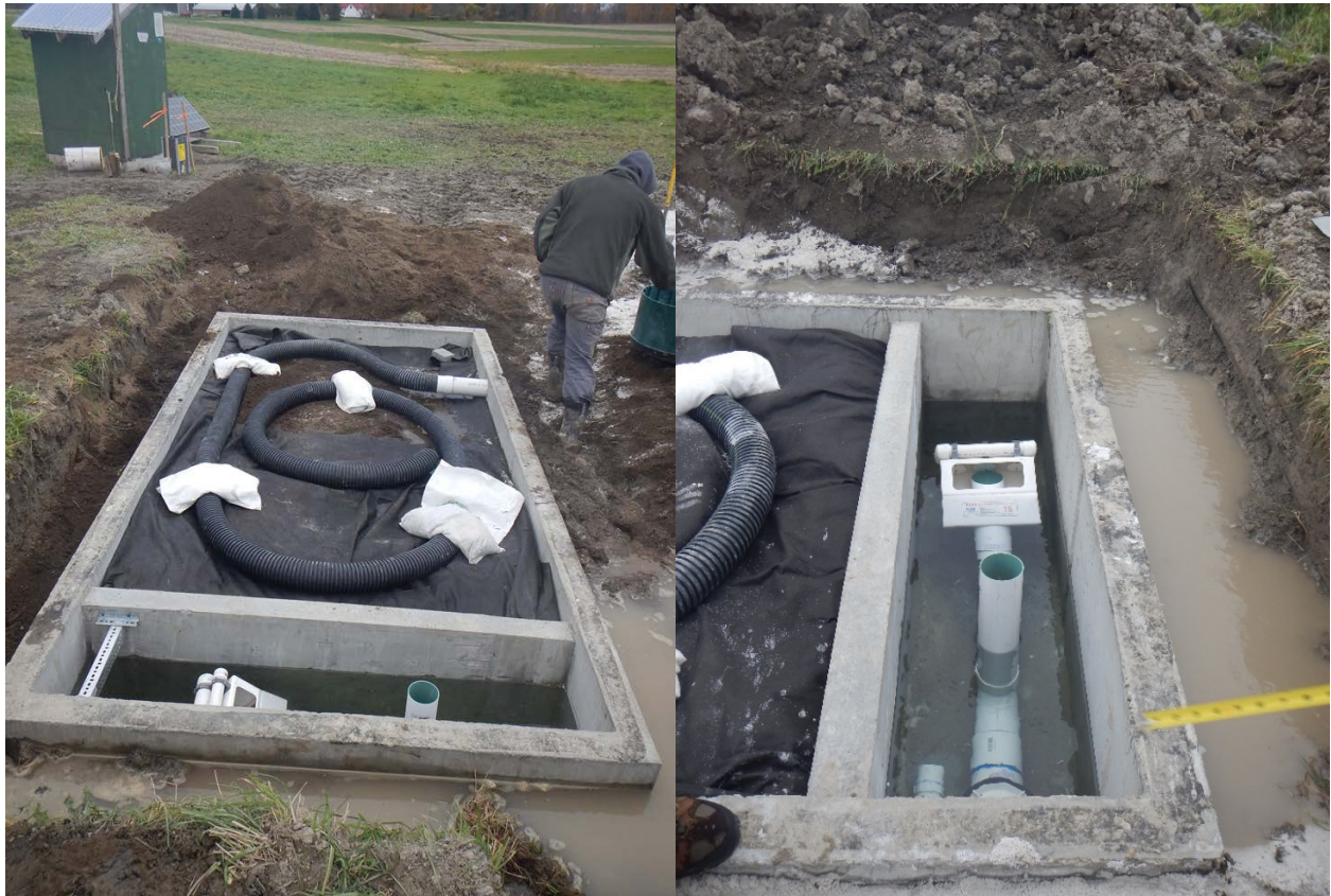
Figure 4: Media (left) and Flout (right) chambers prior to placing lid on Filter A
