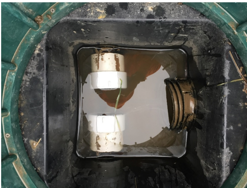
Figure 9. Interior of distribution box
