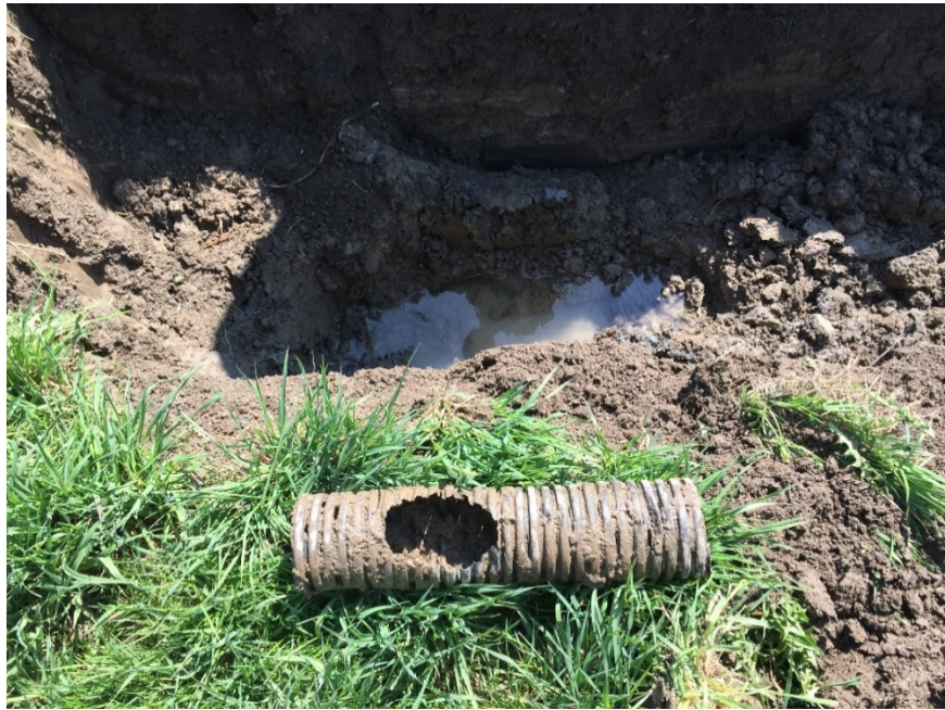
Figure 11: Repair made to tile drain due to a muskrat hole
